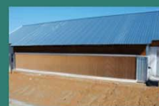
Cooling Pads & Fans
