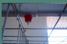
Nipple & PVC Pipe with Saddle
