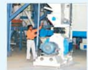
Hammer Mill on Ground Floor
