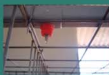
Nipple & PVC Pipe with Saddle
