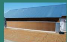
Cooling Pads & Fans
