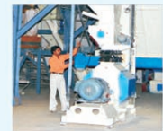
Hammer Mill on Ground Floor
