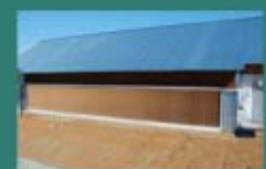
Cooling Pads & Fans
