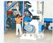
Hammer Mill on Ground Floor
