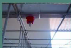
Nipple & PVC Pipe with Saddle
