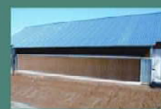
Cooling Pads & Fans
