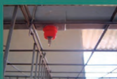
Nipple & PVC Pipe with Saddle
