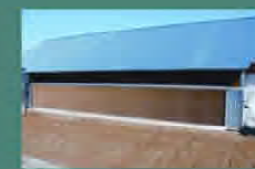
Cooling Pads & Fans
