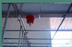
Nipple & PVC Pipe with Saddle
