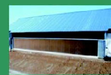
Cooling Pads & Fans
