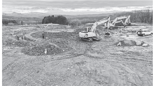
In Sakata on the main island of Honshu, cowsheds are currently being built in addition to the biogas plant. This location should be ready in autumn 2021.
