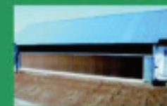
Cooling Pads & Fans
