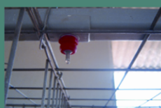
Nipple & PVC Pipe with Saddle
