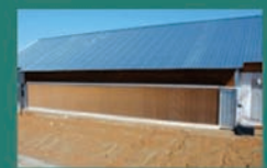
Cooling Pads & Fans
