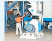
Hammer Mill on Ground Floor
