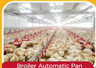
Broiler Automatic Pan Feeding & Drinking System
